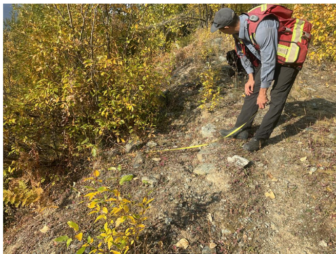
Photo 3: Minor fill settlement at 5.47 km on Rossiter FSR.
